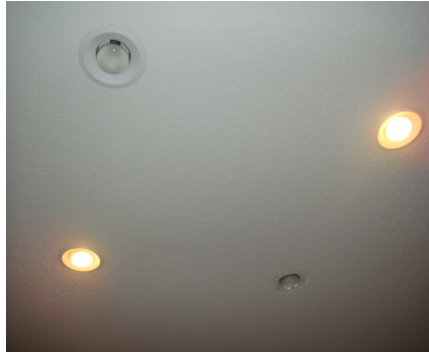
Burnt out light bulbs
