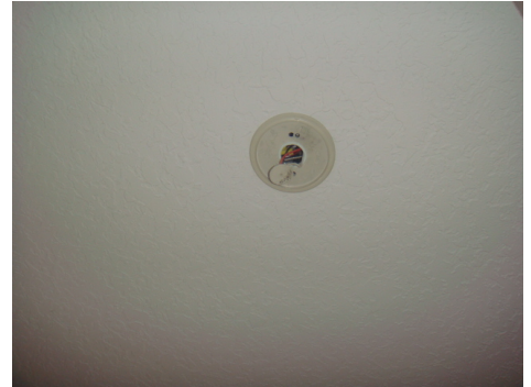
Missing smoke detector
